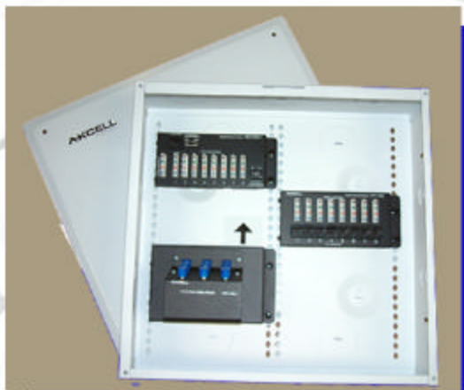
Above: A 14" structure wire panel used to distribute telephone and television signals.
