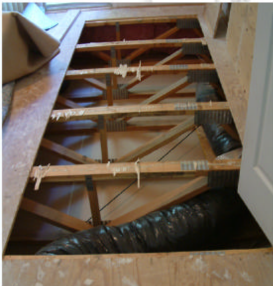
Above: A second story floor opened up to install a projector in a downstairs living room.
